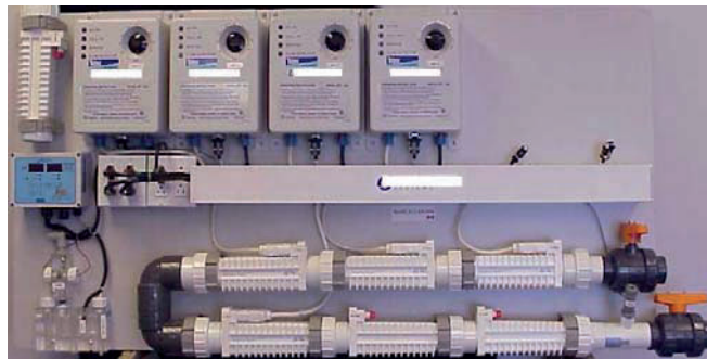
Picture: Control Panel and Electrolytic Cells
