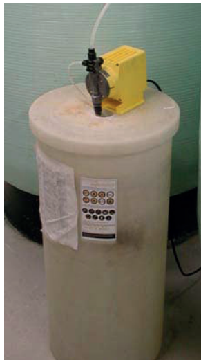
Picture: Sodium Hypochlorite Tank and Hypochlorinator
